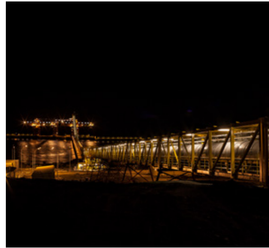
The access bridge is made up by an infrastructure of eighty leaned steel piles anchored to the bottom of the sea. Courtesy of Invierno Mine.
