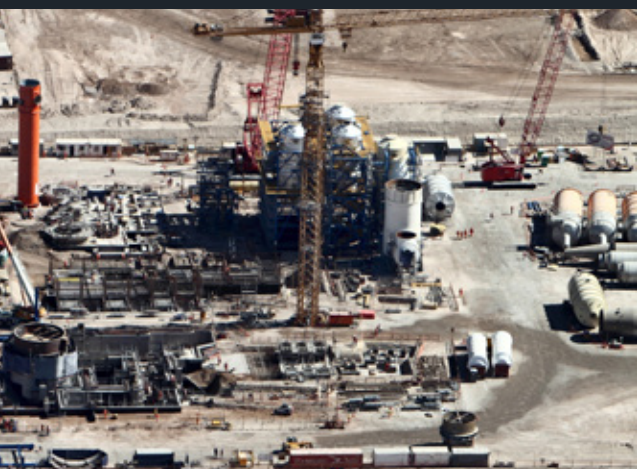
In area 5000 corresponding to the roasting site, calcine hopper buildings were considered, pressurized vessels for pneumatic transport, ecometals, compressors room and two electric rooms. Courtesy of Codelco.
